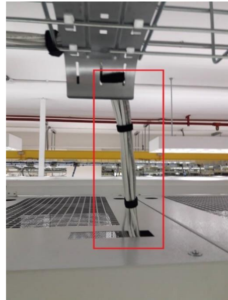
Figure 1.4 Cable dropping from bottom edge of basket
